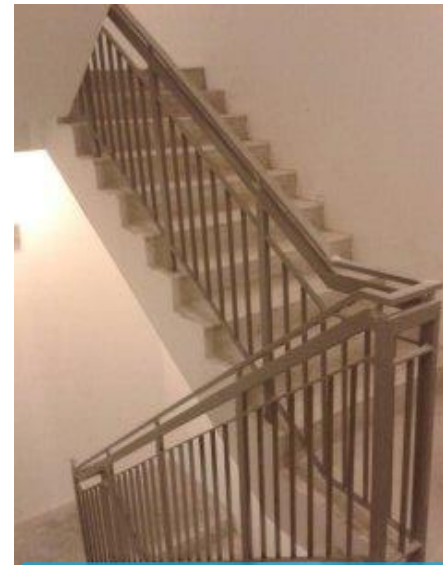
RAILING WITH PAINT
